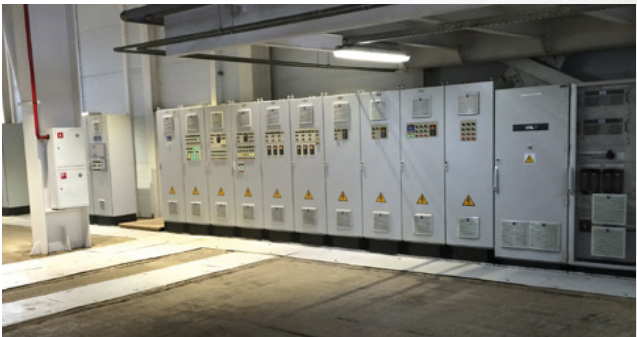
ACS and LVCD of Gas Turbine Plant
